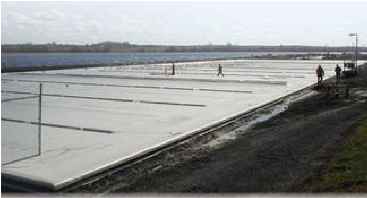
The Casco facility's new GTI floating geomembrane cover
